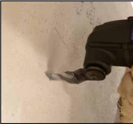
The saw can be used for a variety of jobs, the one above is cutting a socket hole in plaster board.
